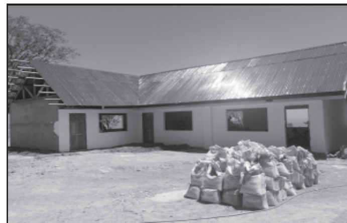
CSR: New community center will be finished this May with a new barangay hall, health clinic and basketball court.
