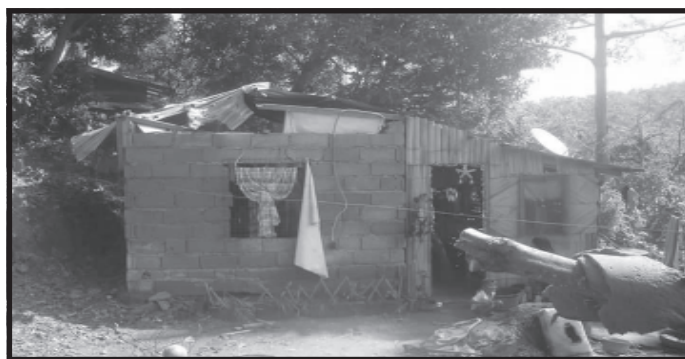
One of the damaged house in sitio Kanluman
